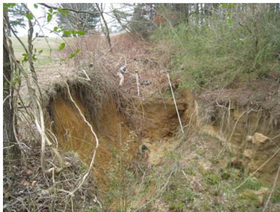
Figure 1: Damage to channel caused by stormwater erosion. Photo credit: Center for Watershed Protection
